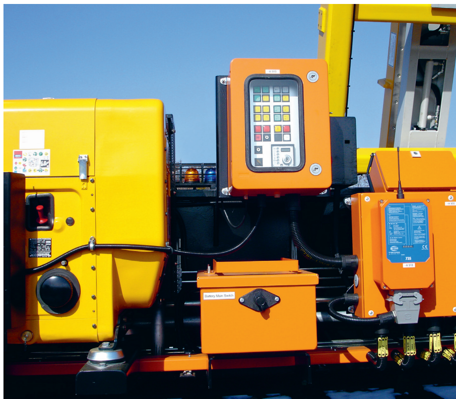
↑ Diesel engine and local control panel
